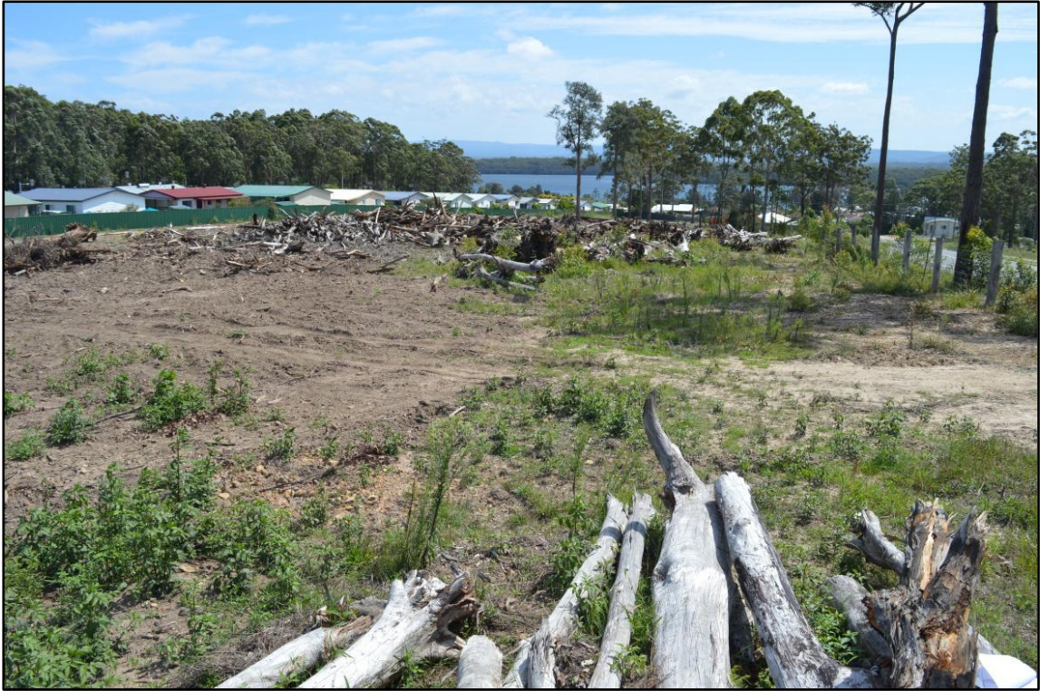
Plate 1: View looking west across Lot 6 on the southern side of Anson Street.
